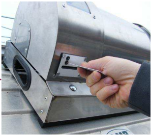
“Gate” system with electronic control
